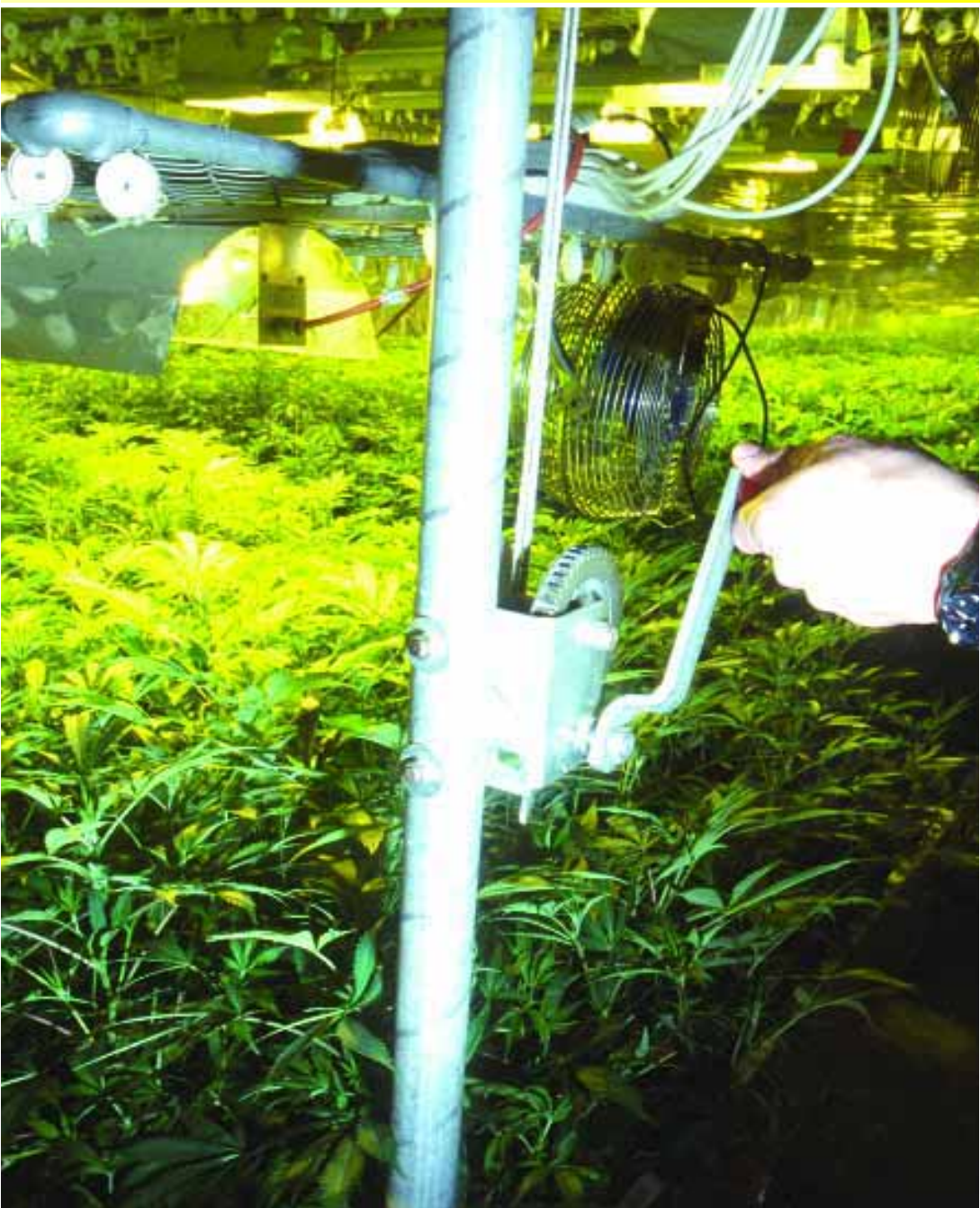
A single handle raises and lowers an entire roomfull of lights!
